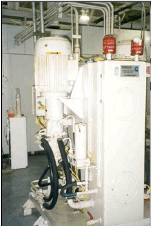
Figure 5 Engine manufacturer Cummins replaced 296 motors ranging from 1 to 125 hp with premium-efficiency versions at its Midrange Engine Plant in Walesboro, Indiana. Although the new motors were only a few percent more efficient than the standard motors they replaced, they reduced power costs by $80,000 per year.
