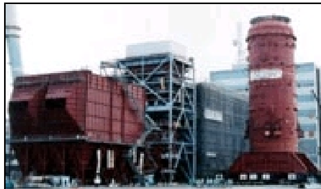
Figure 1 The boiler installed at the Karita Power Station of Kyushu Electric Power Co. in Japan. Burning coal with pressurized fluidized bed combustion (PFBC), the plant operates at 42.8 efficiency, compared to an average of about 34 percent in the U.S. An older PFBC in Stockholm has run since 1991 at about 90 percent efficiency, because it uses heat from the exhaust to warm offices, homes and stores. (Source: IHI Industries.)
