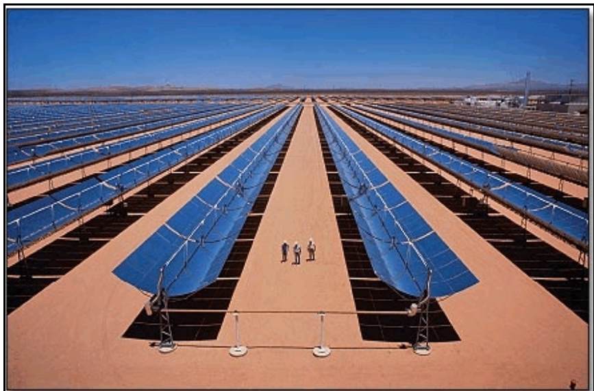
Figure 13 The largest 'solar thermal-electric' installation in the world, the Luz project in California's Mojave Desert, has a peak output of some 350 MW, or about 350,000 homes. It has been making zero and near-zero polluting electricity since the 1980s.
