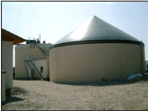
Figure 5 Location: Fakler, Germany Year: 2005 Input: Corn, grass and wheat silage Digester: Concrete tank, 1 045 m 3 Co-generator: Gas engine 250 kW Designer: Krieg & Fischer
