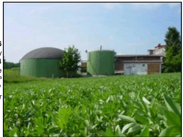
Figure 6 Location: Hofgut Holland, Germany Year: 2004 Input: Pig dung, turkey dung, grass and corn silage Digester: Concrete tank, 350 m 3 Co-generator: Gas engine 60 kW Designer: Krieg & Fischer
