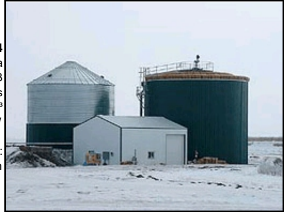
Figure 4 Location: Saskatoon, Canada Year: 2003 Input: Manure, potatoes Digester: Steel tank, 2 000 m 3 Co-generator: Micro turbine, 4 x 30kW Designer: Krieg & Fischer Source of this and following items: Electrigaz, http://www.electrigaz.com/company_en.htm
